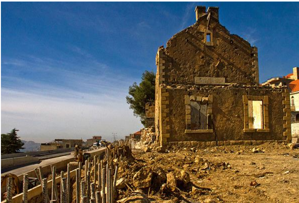
The former station at Bhamdoun, a mountain village between Beirut and the summit at Dar Al Baidar, is now being destroyed by the construction of the new express highway beside it.
